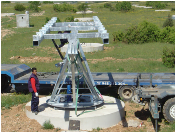
Frame with crossbeams over the central body of the tracker.
